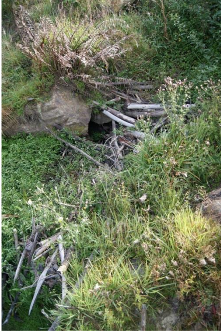
Figure One - The culvert on the south east end of the creek must be kept clear for water flow and any spawning activity of fish in the area.
